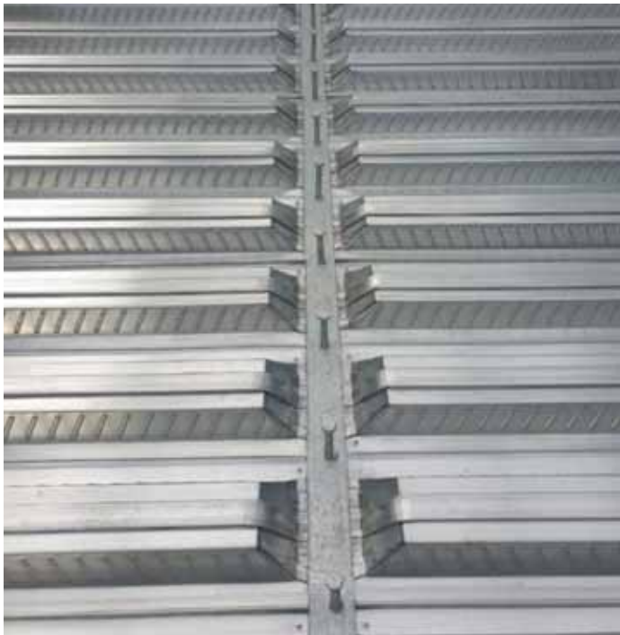
Figure 4: Discontinuous decking with crushed ends (courtesy of Kingspan)
