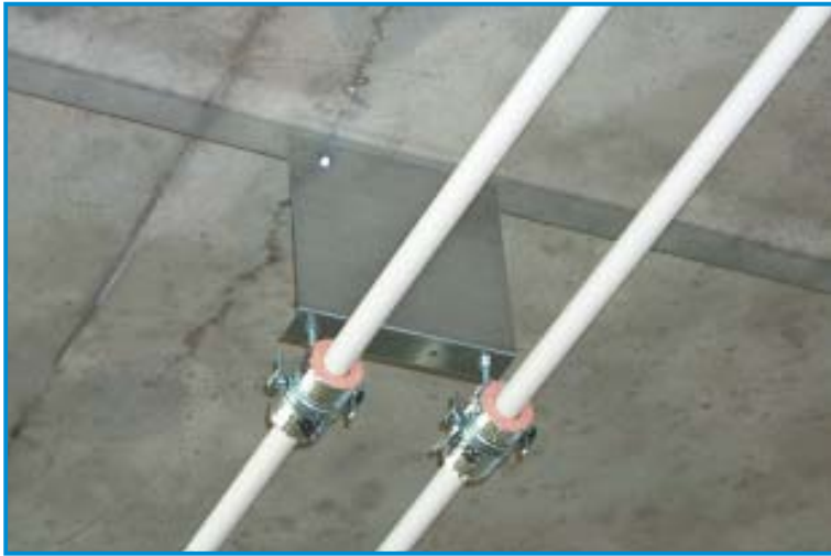
Figure 15: Chilled water pipework suspended from a sheet-metal bracket installed by a ceiling contractor.
