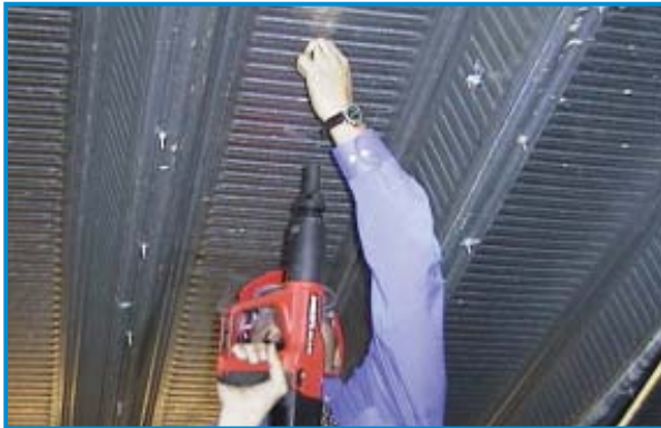
Figure 10: Powder-actuated fastening (otherwise known as shot firing) is suitable for many types of structural slab.
