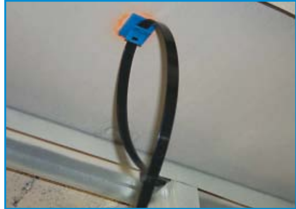
Figure 11: adhesive fasteners are ideal for supporting lightweight services. ©BSRIA.
