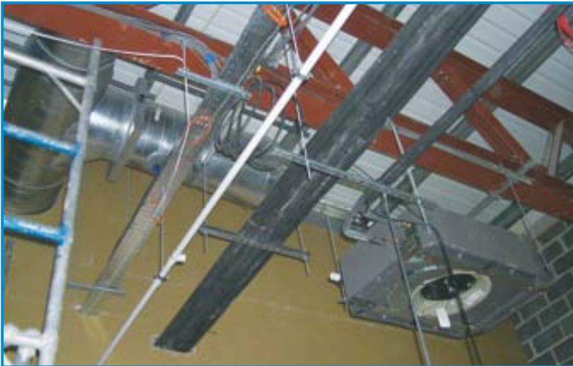
Figure 3: The suspension of different services from the structural steelwork is often improvised by multiple trades passing through the same area. This can create conflict and delays, and increase the costs of the project.
