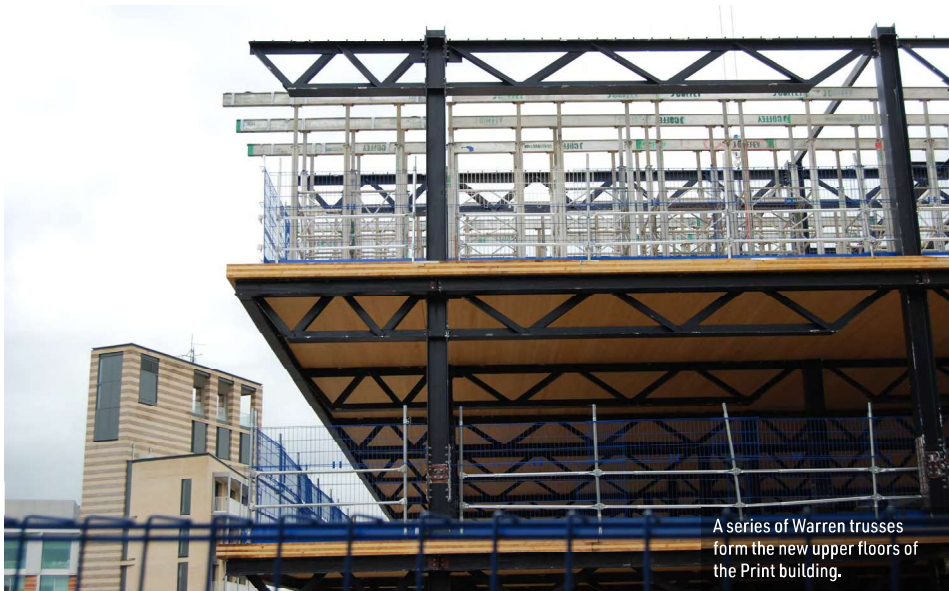
The existing Print building has been remodelled and the areas highlighted in pink were demolished prior to the new steelwork being installed.
