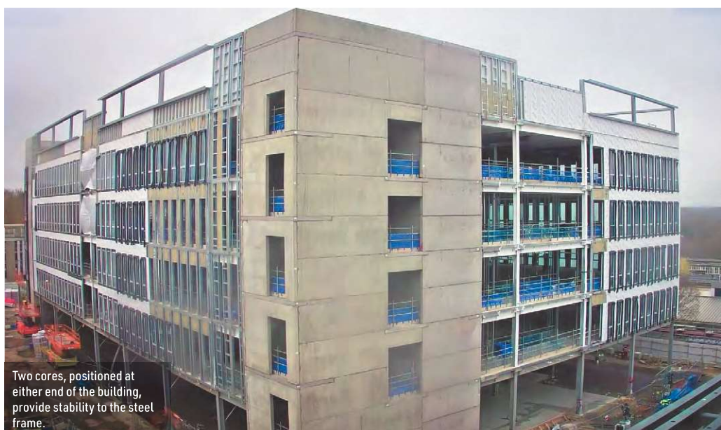
Finishing touches are applied to the façades in readiness for this month's opening.
