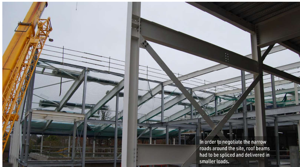
Part of the steel frame was omitted until a second phase, which allowed the cladding to be installed from within the site's footprint.
