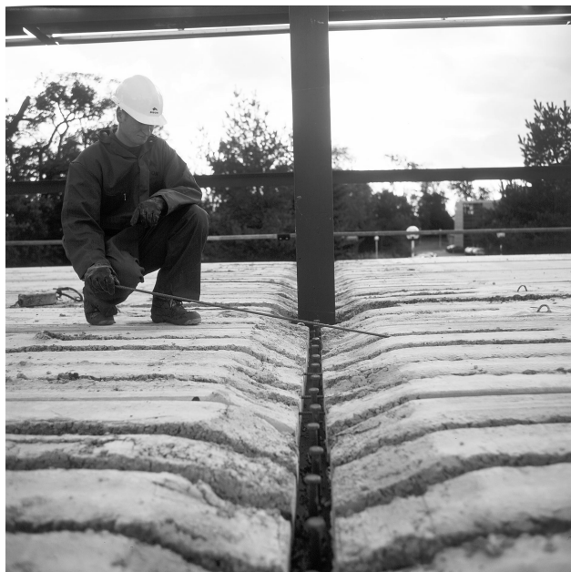
Figure 4.14 composite floor construction with precast concrete hollow core units, showing transverse reinforcement bars placed within open cores
