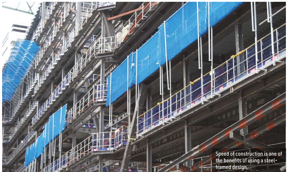
Cellular beams, accommodating the building services, are used throughout the project.
