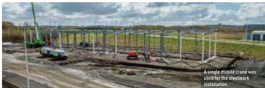
A ground improvement programme was undertaken prior to the steel erection beginning.
