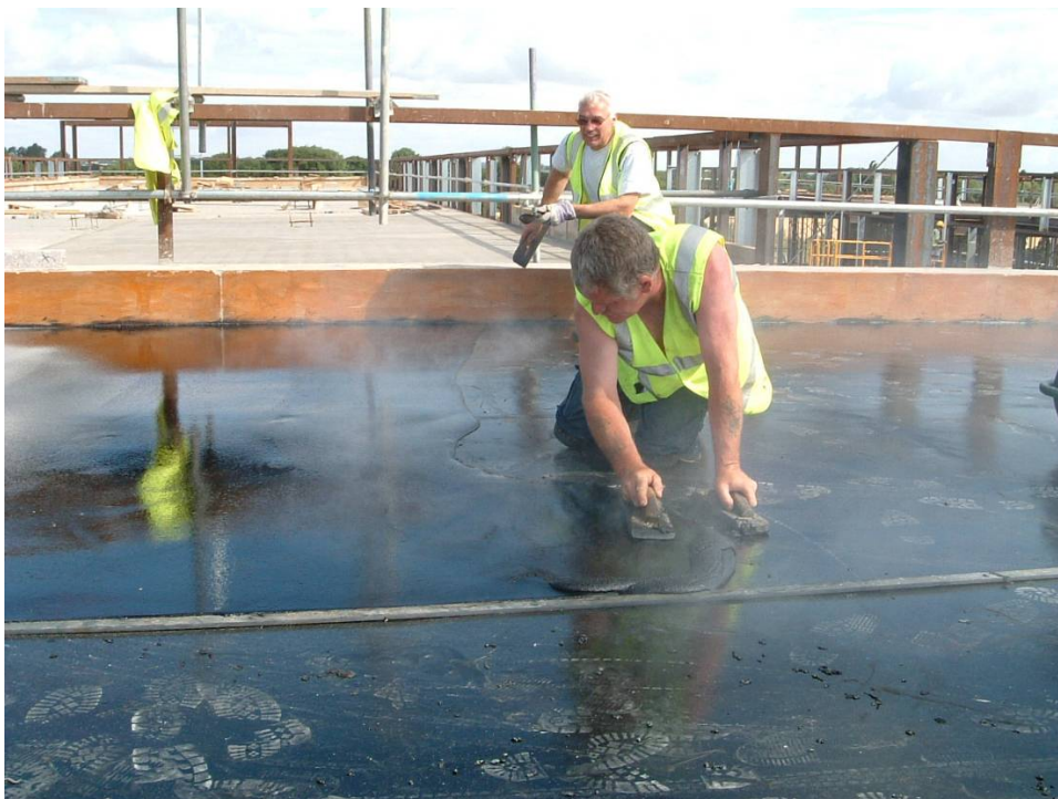
Figure 3.6 Mastic asphalt be laid over a sheathing felt and glass tissue faced polyurethane boards which were first bonded in hot bitumen onto a felt vapour control layer (Photograph by kind permission of Permanite Asphalte)
