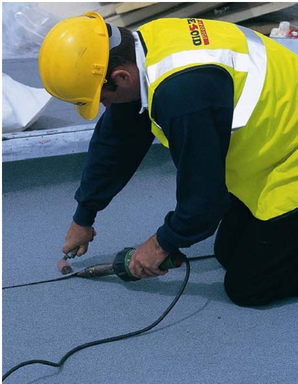
Figure 3.4 A built up bituminous membrane being sealed by hot air welding (Photograph by kind permission of Ruberoid)
