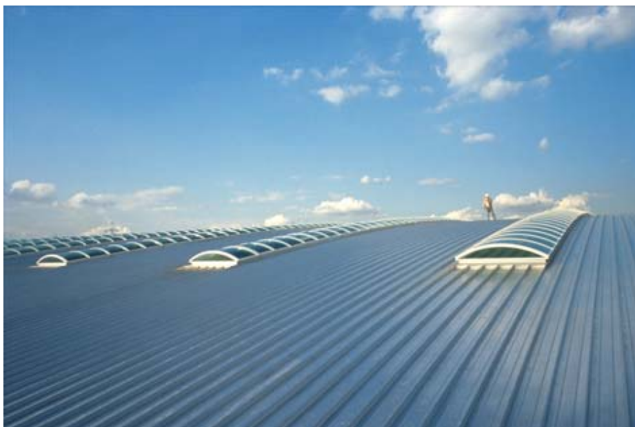
Figure 2.12 Standing seam or secret fix sheeting (Photograph by kind permission of Wilkinson Eyre Architects. Photographer Morley von Sternberg)
