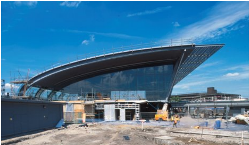
Figure 2.13 A curved roof using a standing seam system (Photograph by kind permission of Wilkinson Eyre Architects)
