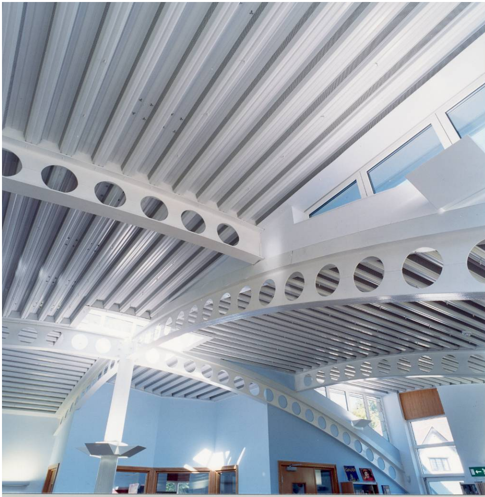
Figure 2.6 Standing seam roof over a perforated structural support deck with mineral wool insulation to provide sound absorption in a library (Photograph by kind permission of Corus P &P)
