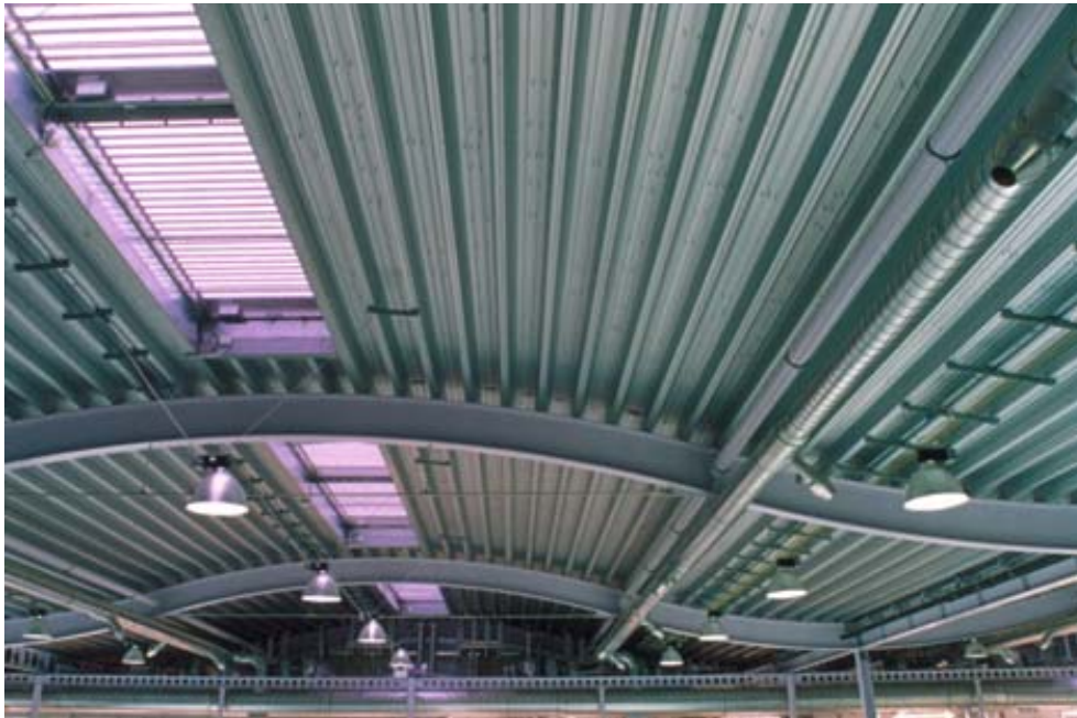
Figure 3.3 Roof decking with a deep profile fixed between the main frame work with minimal support from secondary steel work. (Photograph by kind permission of Wilkinson Eyre Architects. Photographer Paul Rapson)
