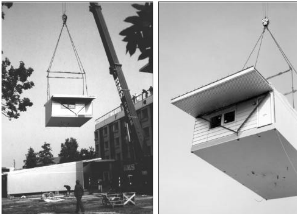
Figure 11.4 Erection of modular units in roof-top extension in Copenhagen (see completed building in Figure 4.4)
