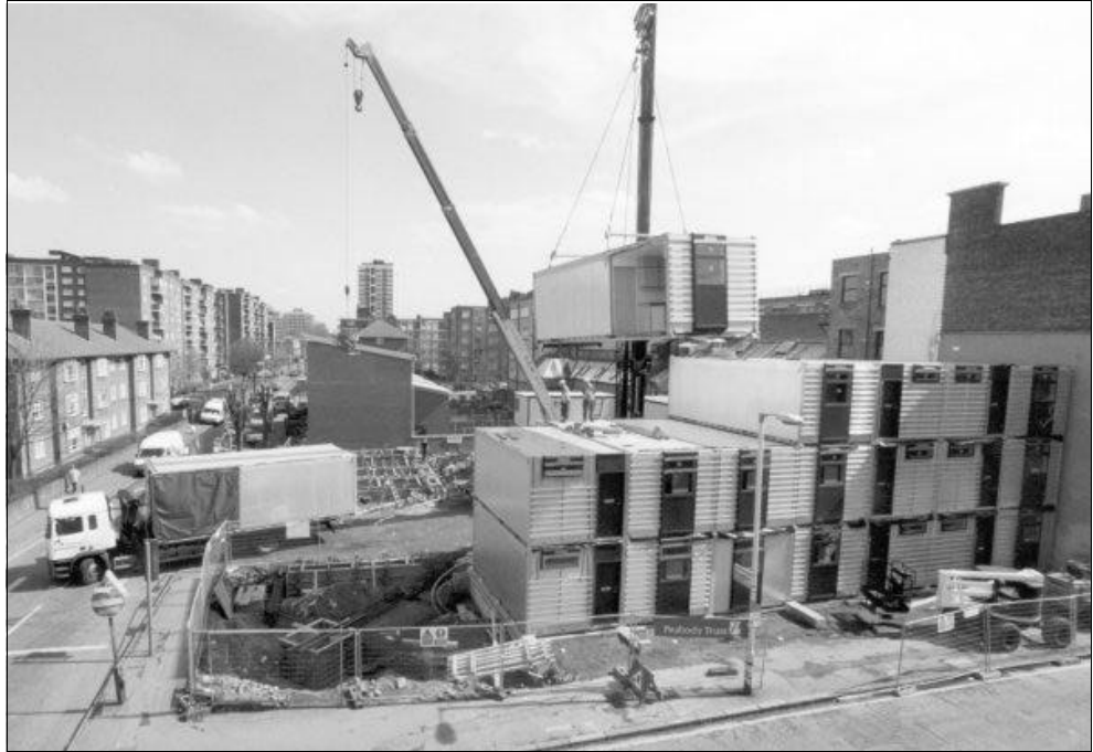
Figure 5.7 Installation of Yorkon module at Murray Grove, Hackney (see artist's impression of completed building in Figure 3.3)
