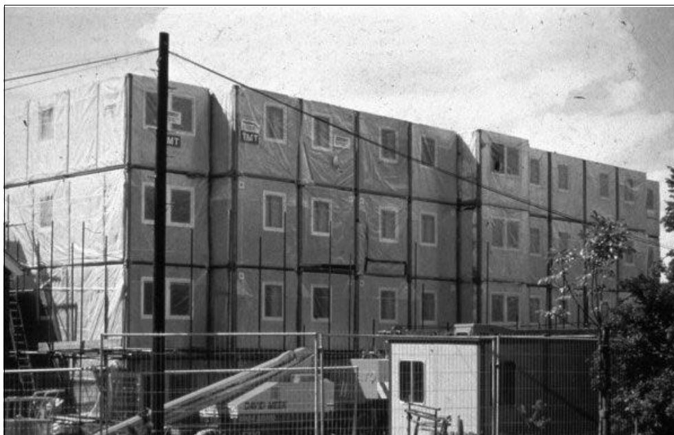
Figure 3.2 Modular units used in the student residence at the University of Wales, Cardiff (see completed building in Figure 1.1)
