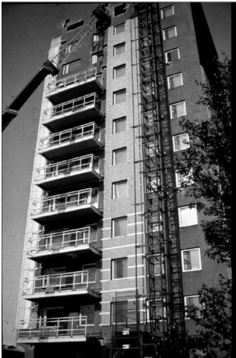
Figure 11.6 Conversion of an apartment block in Finland showing new balconies and over-cladding
