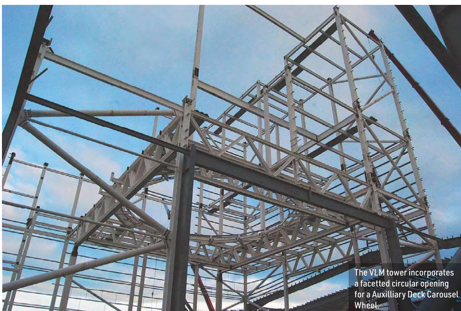
The five-storey CCV tower was one of the final steel elements to be erected.
