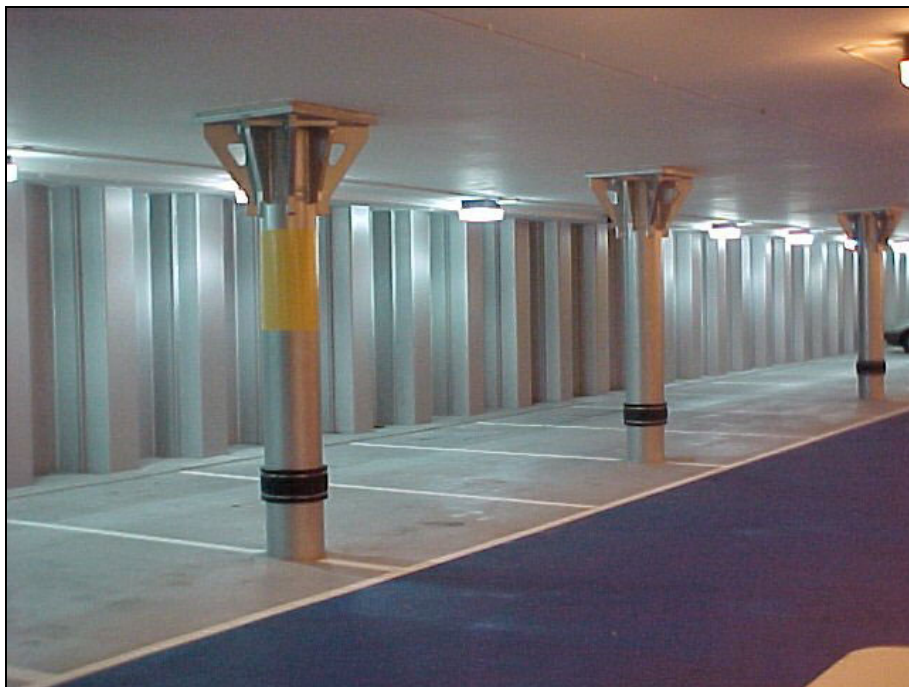
Figure 7.2 Millennium Car Park, Bristol showing sheet piling and the column head detail supporting the floor slab
