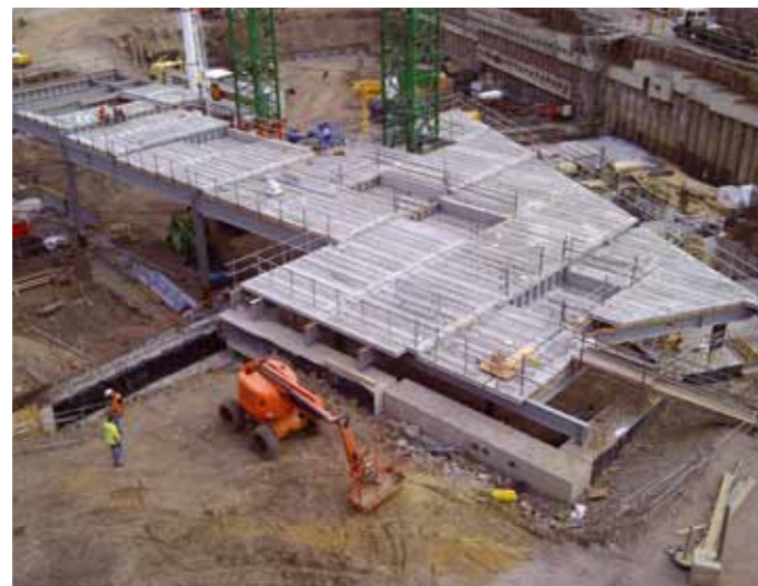
About 600 tonnes of steel was erected in eight weeks to create the podium
