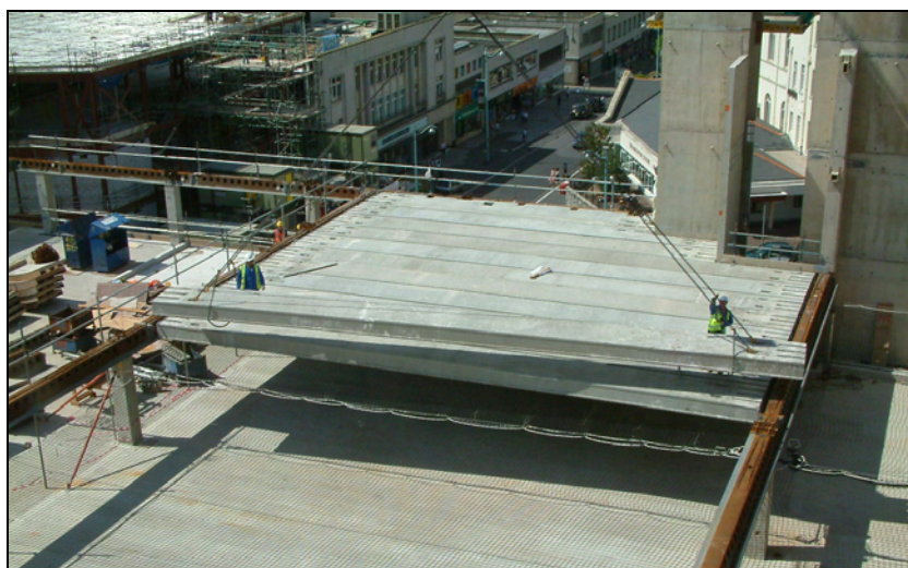
Figure A.7 Precast floor units at Drake Circus shopping centre, Plymouth
