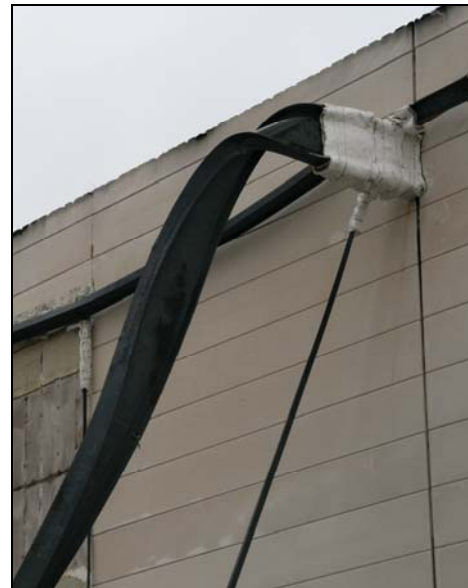
b) Partially fire protected steel beam crossing a fire wall fixed to steel columns
