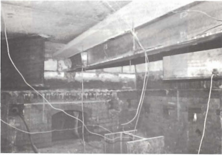
FLOOR BEAM WITH INDICATIVE BEAMS BOLTED TO THE UNDERSIDE OF THE FURNACE ROOF FIG. 22
