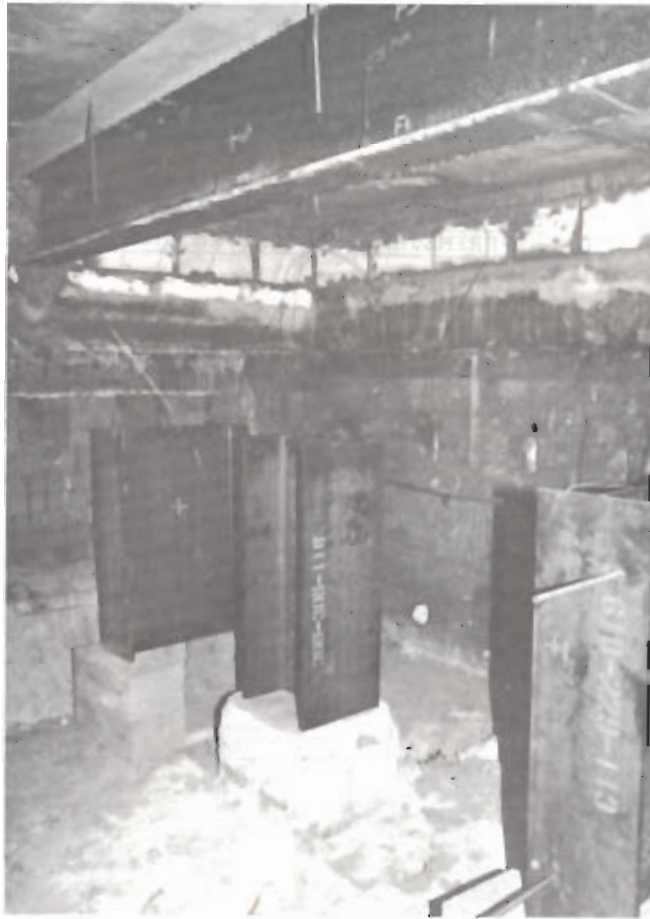
INDICATIVE COLUMNS PLACED ON PLINTHS ON THE FLOOR OF THE BEAM FURNACE FIG. 23
