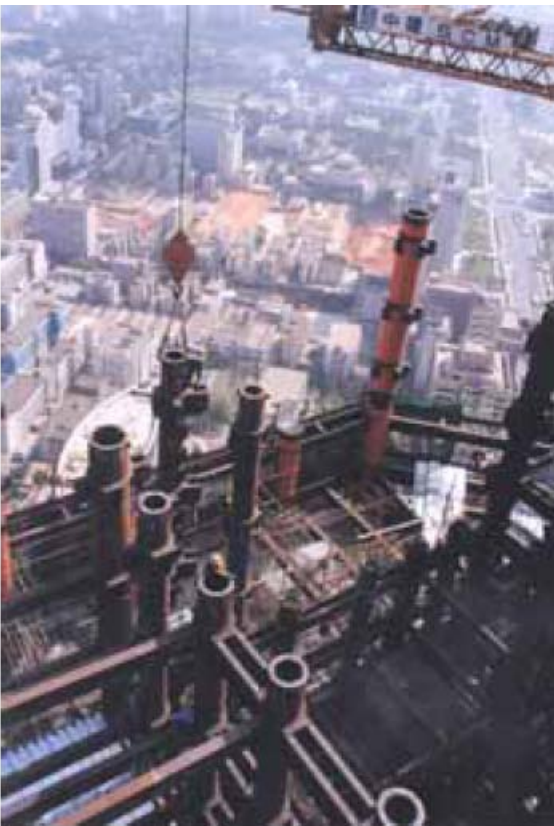
Figure 1-8 SEG Plaza under construction (photo courtesy of Prof. L H Han, Tsinghua University, China)
