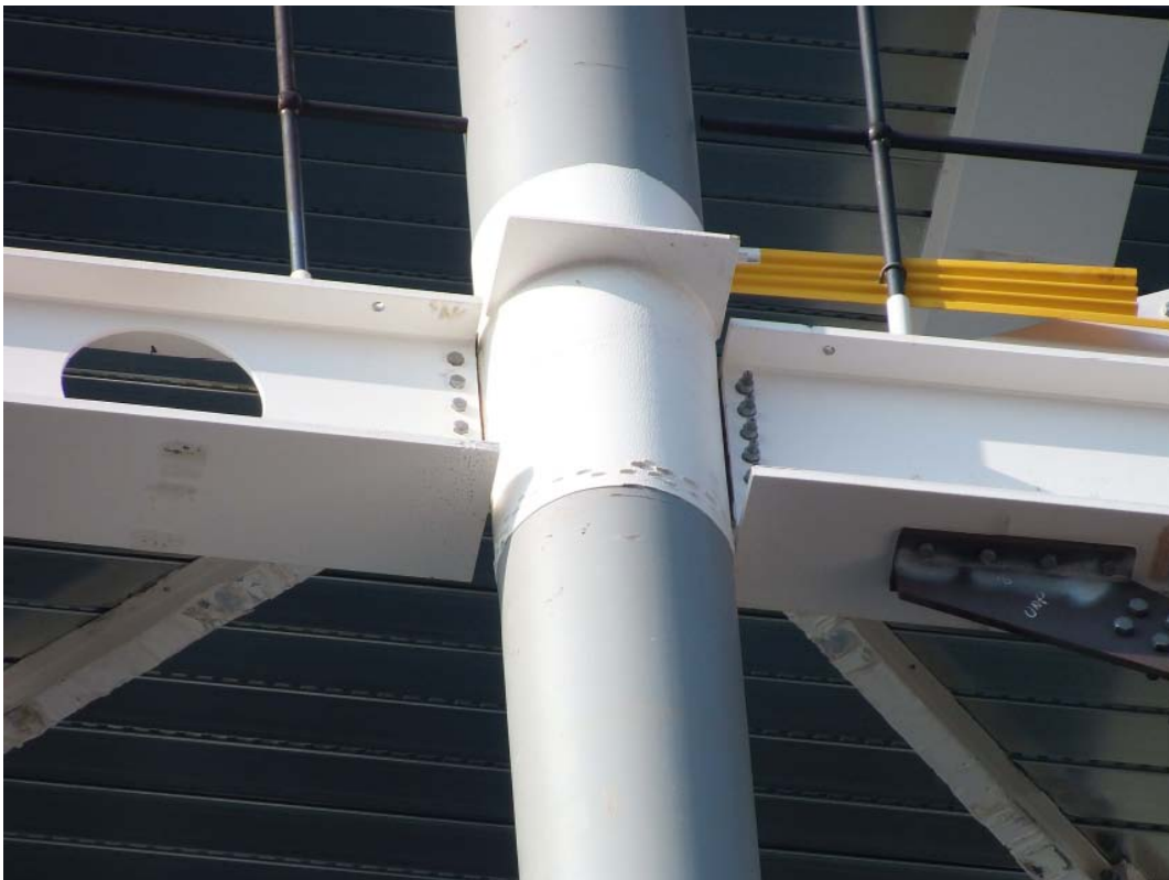
Figure 1-11 Exposed concrete filled sections
