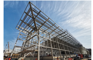
Right: The roof truss was fabricated on the ground and lifted into place
