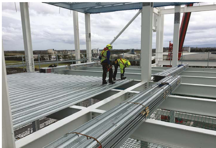
Figure 1: Bundles of decking positioned on the structure and the individual sheets then installed by hand (Photo courtesy of Severfield)
