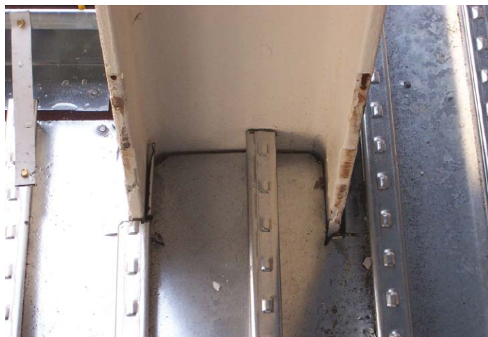
Figure 2: Typical detail of decking installation around a column (Photo courtesy of SMD)
