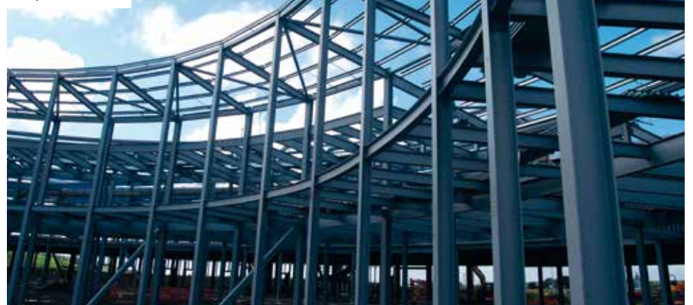
A combination of faceted straight members and curved beams form the courtyards
