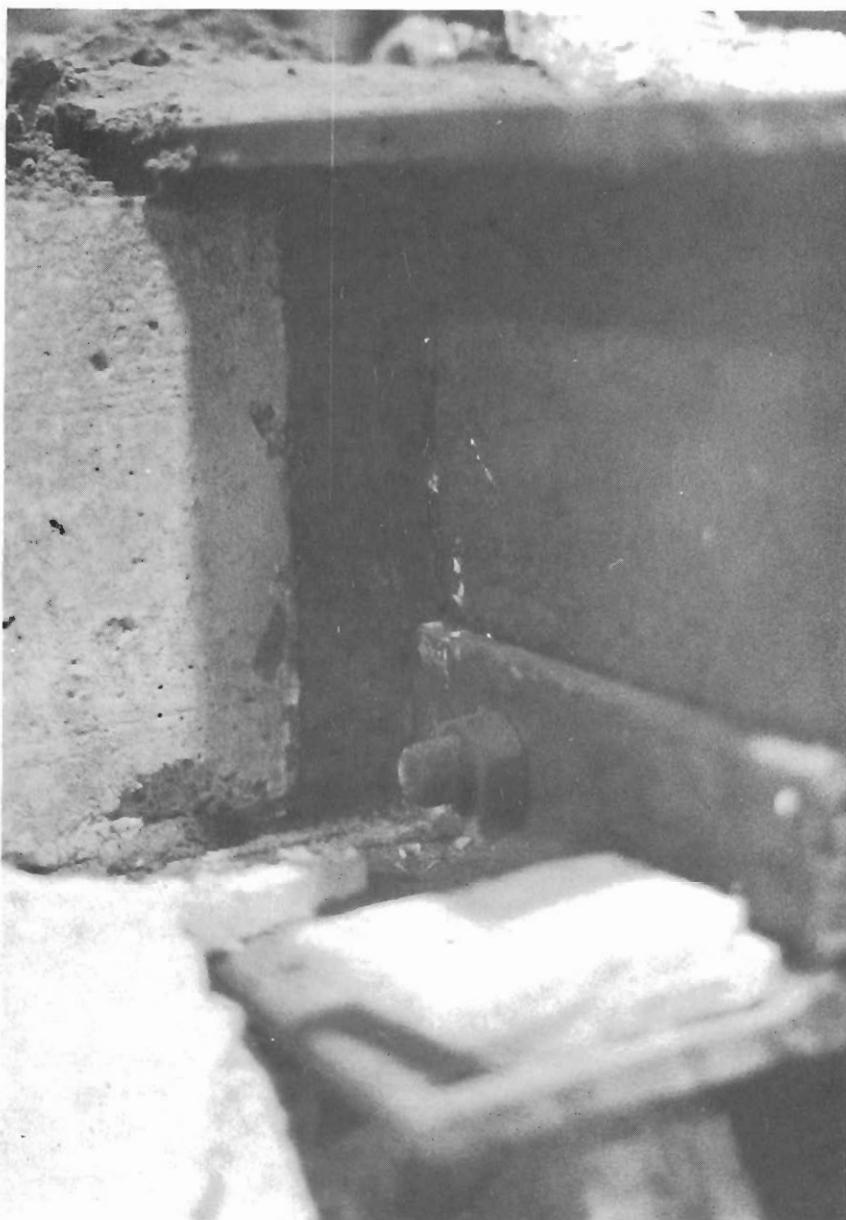
VOID FILLED WITH SAND TO SIMULATE THE THERMAL CHARACTERISTICS OF THE SCREED USED IN SITE PRACTICES
