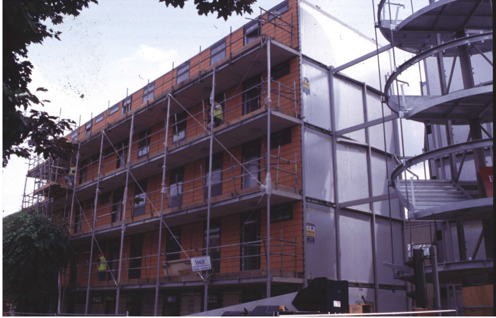
Figure 1.1 Murray Grove in London for Peabody Trust using prefabricated steel framed modular units manufactured by Yorkon Ltd
