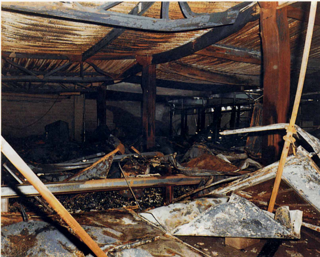
Plate 8: View towards Exchange Square and Phase 7 wall showing deformation of the structure. Note: a) The deformed cols. C32, C33 and C34. b) The deformed diagonal bracing members of trusses CD5 and CD6 c) The buckling of the lower flanges of beams AC5 and C3 at the column connections.
