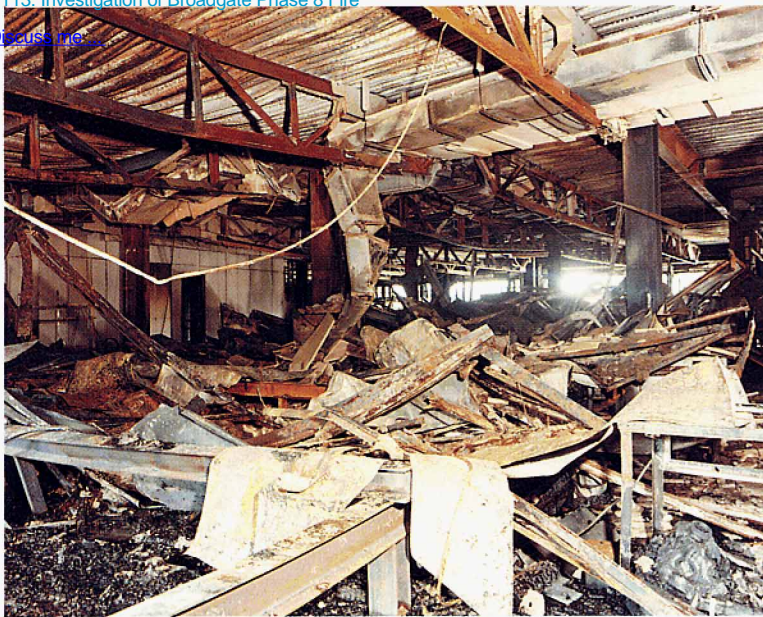
Plate 4: Fire damage to the hut. View towards core and Bishopsgate showing cols. D32, D33 and D34.
