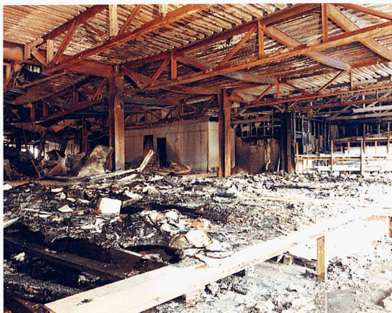
Plate 5: Fire damage to the hut. View from Bishopsgate towards core showing cols. E33 and E34. Note the charred timber joists and the combustible goods unburnt at this end of the structure.
