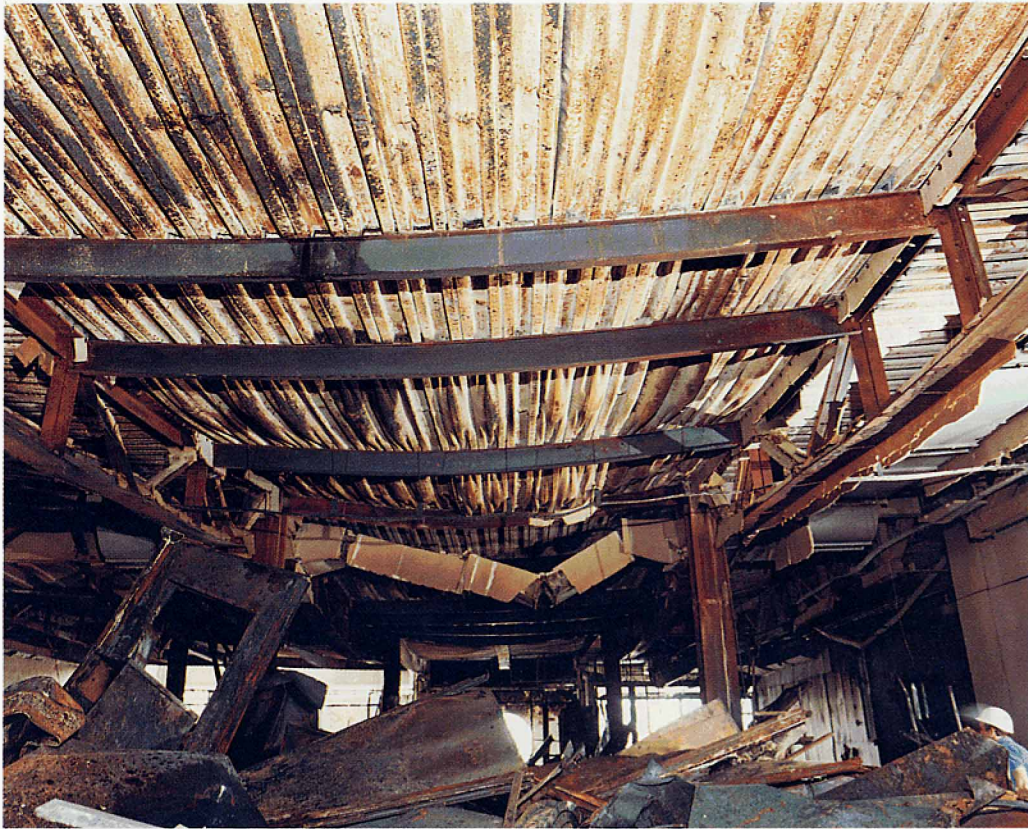
Plate 9: View between lines 33 and 34 facing Exchange Square showing deformation of the structure.
