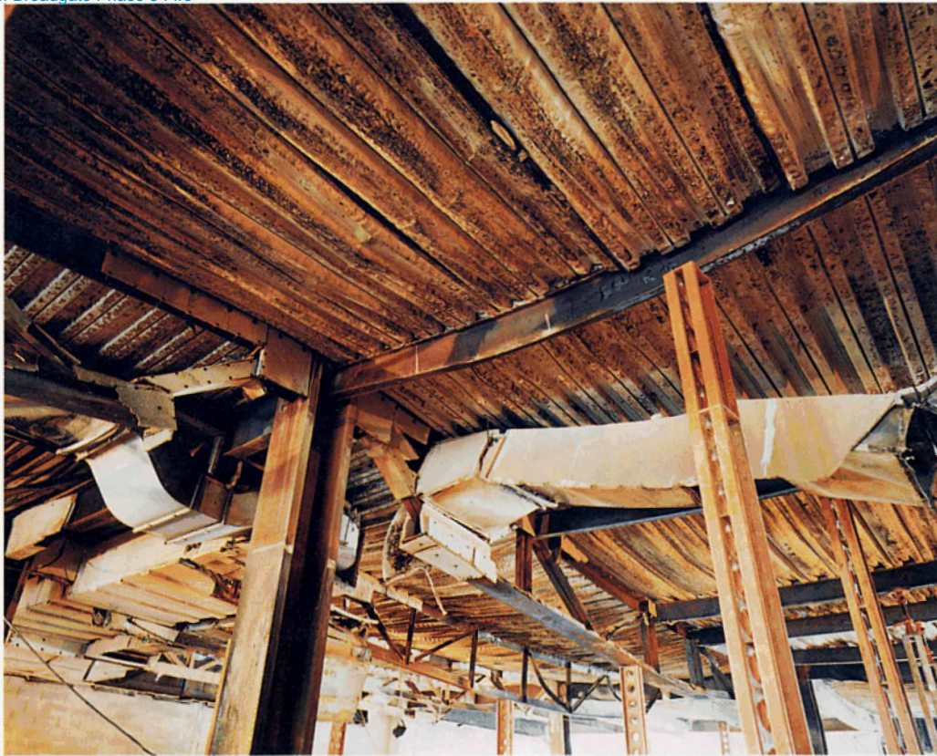
Plate 7: View towards Exchange Square and Phase 7 wall showing damage to the structure. Note: a) The undeformed heavy col. D33. b) The deflection of the light beam D3. c) The detachment of the metal deck from the top flange of beam D3. d) The deformation of truss CD5.
