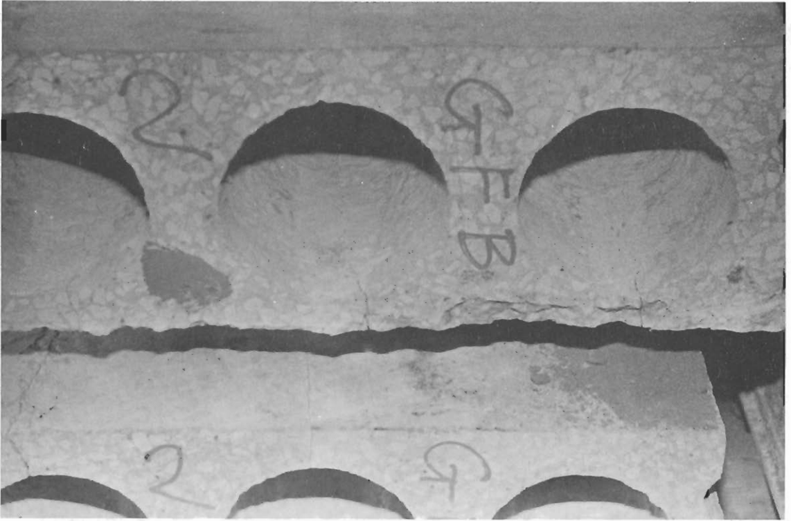
Longitudinal hairline cracks
