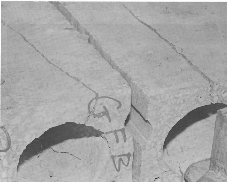
Longitudinal shear cracks
