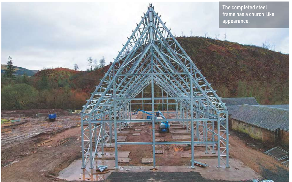
All of the steel trusses were delivered to site as fully-welded sections.
