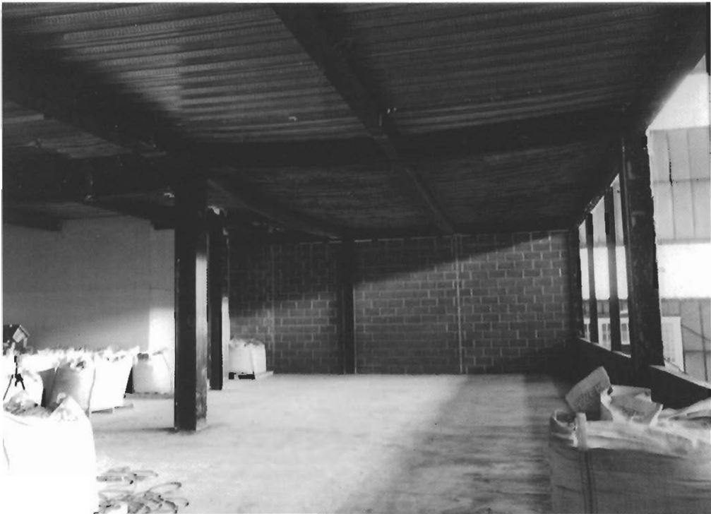
Figure 6.19 Structural deformation following the fire
