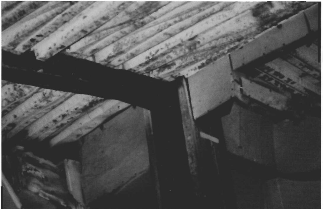
Figure 2.2 A buckled beam and floor slab at Broadgate following the fire
