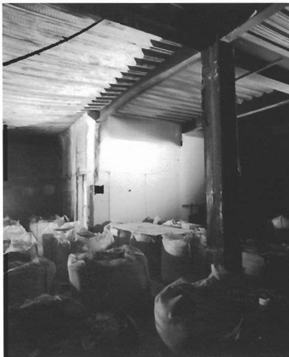
Figure 6.32 Distortional buckling of the beam above the compartment wall (after removal of the wall)
