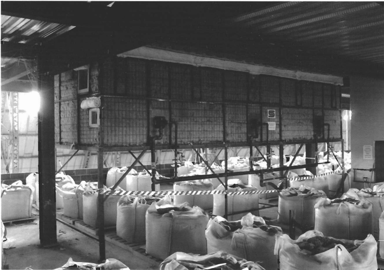
Figure 6.2 Purpose built gas fired furnace
