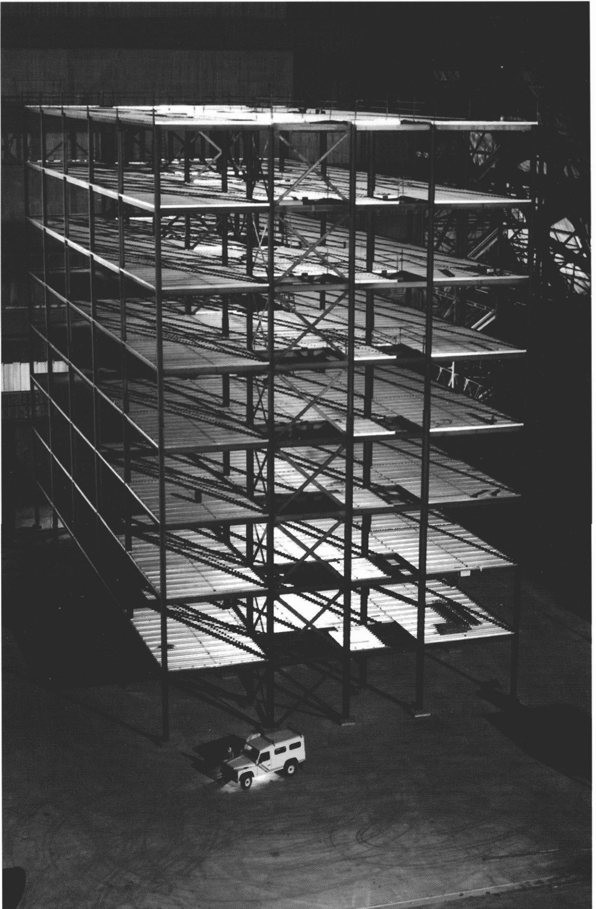
Figure 1.2 General view of test structure illustrating the steel frame and steel decking prior to placing concrete and constructing walls.
