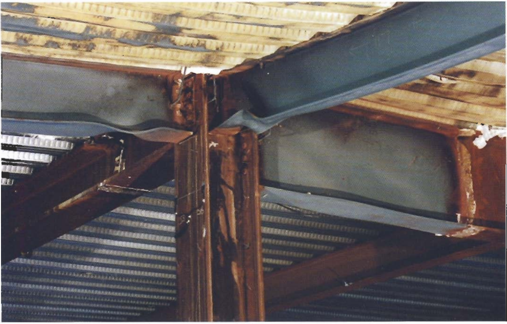
Figure 6.20 Extensive local buckling occurred in the proximity of the beam to column connections
