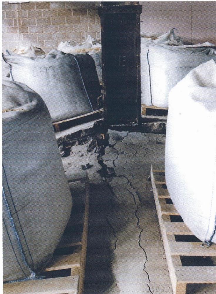
Figure 6.46 Cracking of the composite slab around internal column
