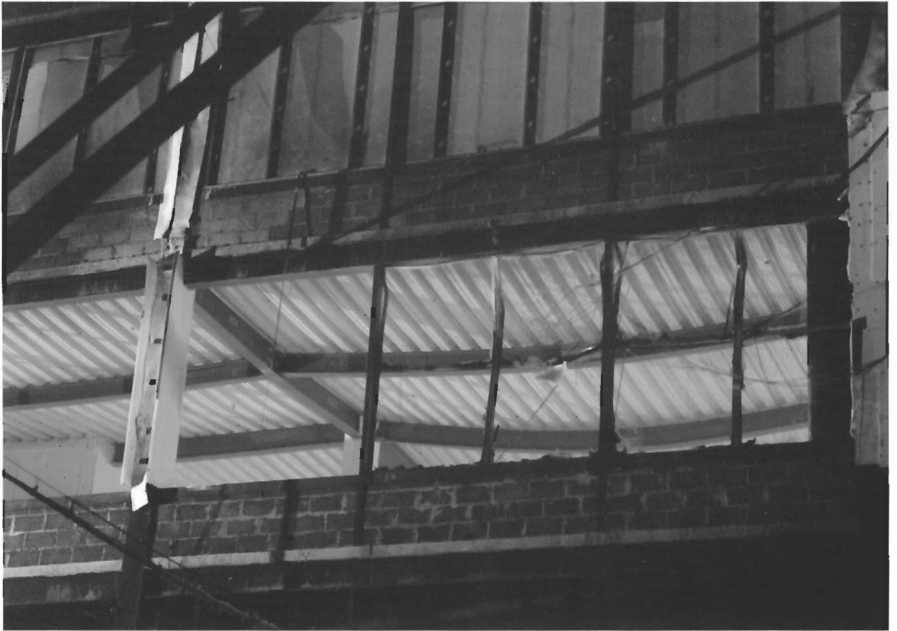
Figure 6.37 Structural behaviour towards the end of the test (notice the local buckling on the second internal secondary beam)
