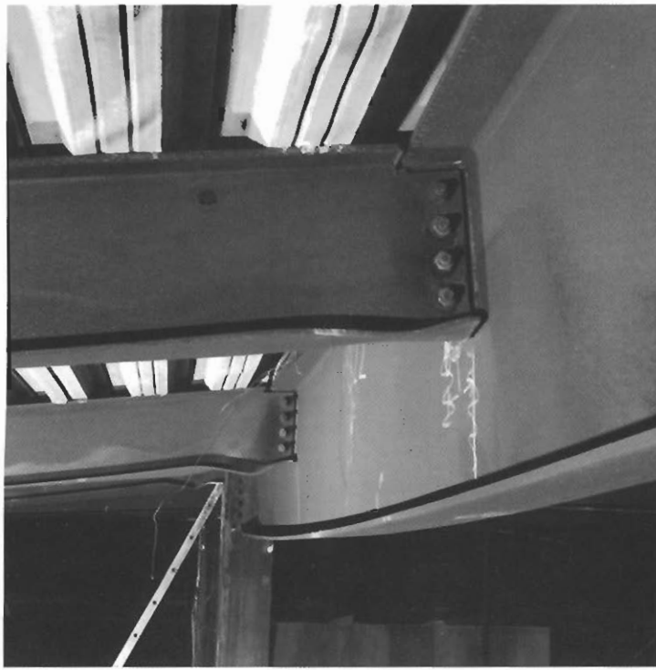
Figure 6.38 Local buckling in the proximity of the steel-to-steel connections
