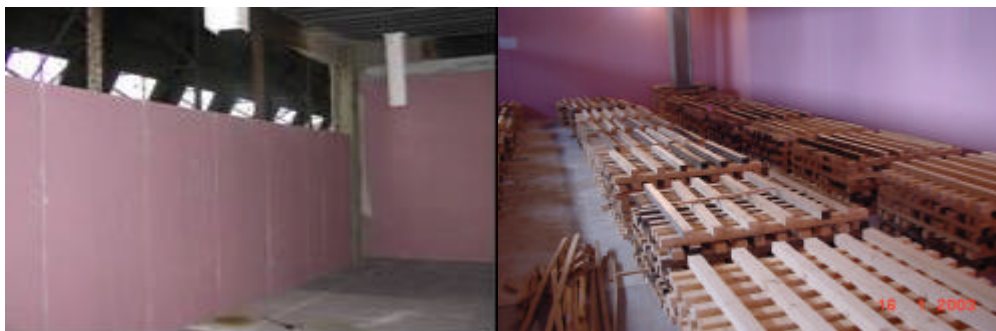
Figure 5 Restricted ventilation and fire load
