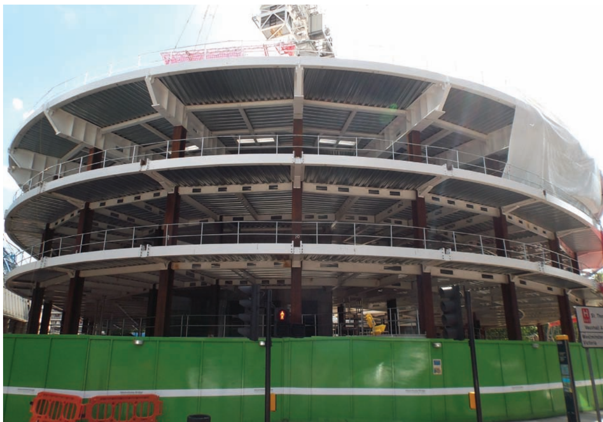
Above The radial steel structure of the sixth form college at the base of the tower.
