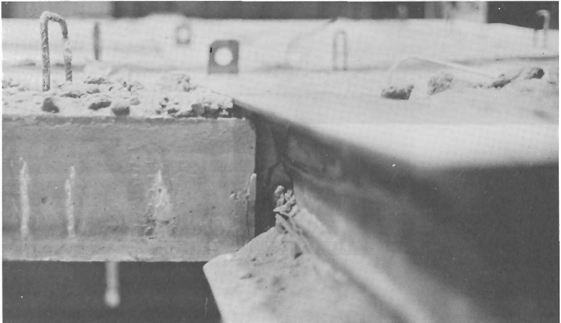
VERTICAL CRACK FORMATION EXPERIENCED BY SOME OF THE CONCRETE SLABS
