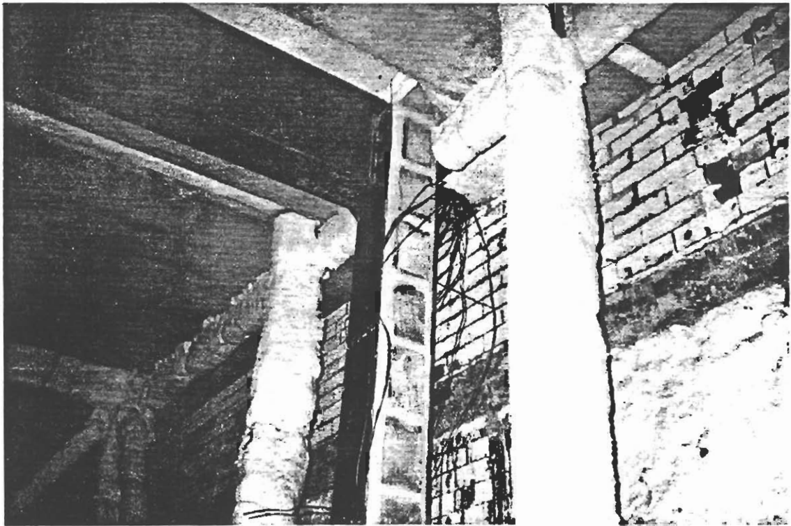
LOADING AND SECONDARY STEEL FRAME LAGGED WITH CERAMIC FIBRE BLANKET
