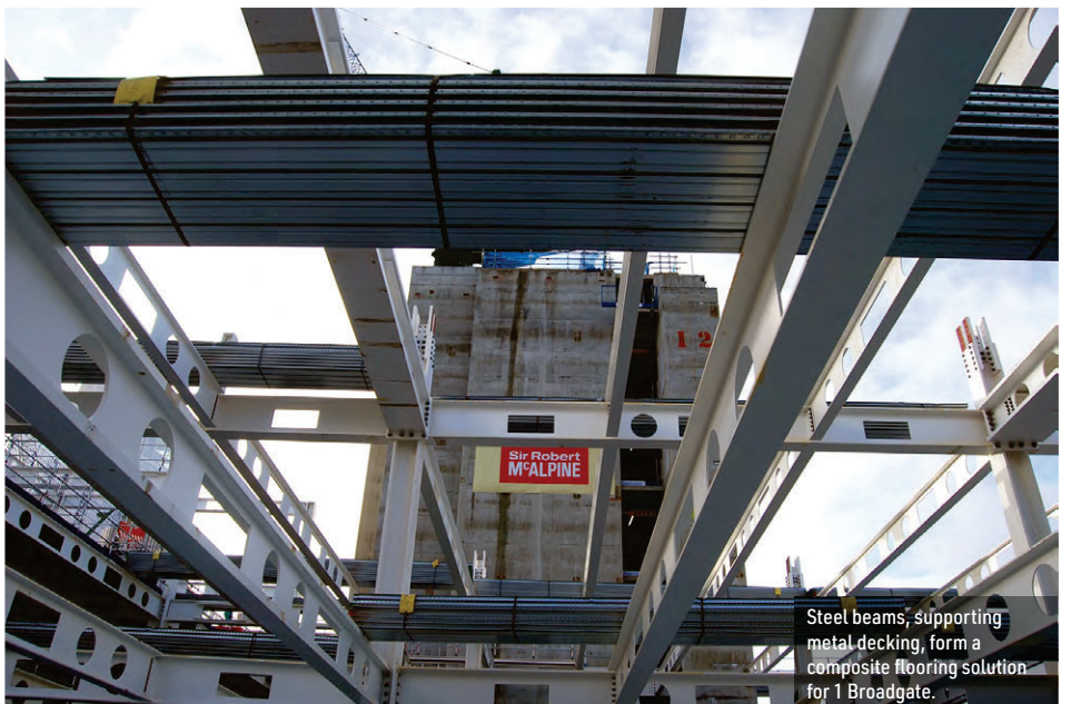
Long span cellular beams, accommodating services, have been used throughout the scheme.
