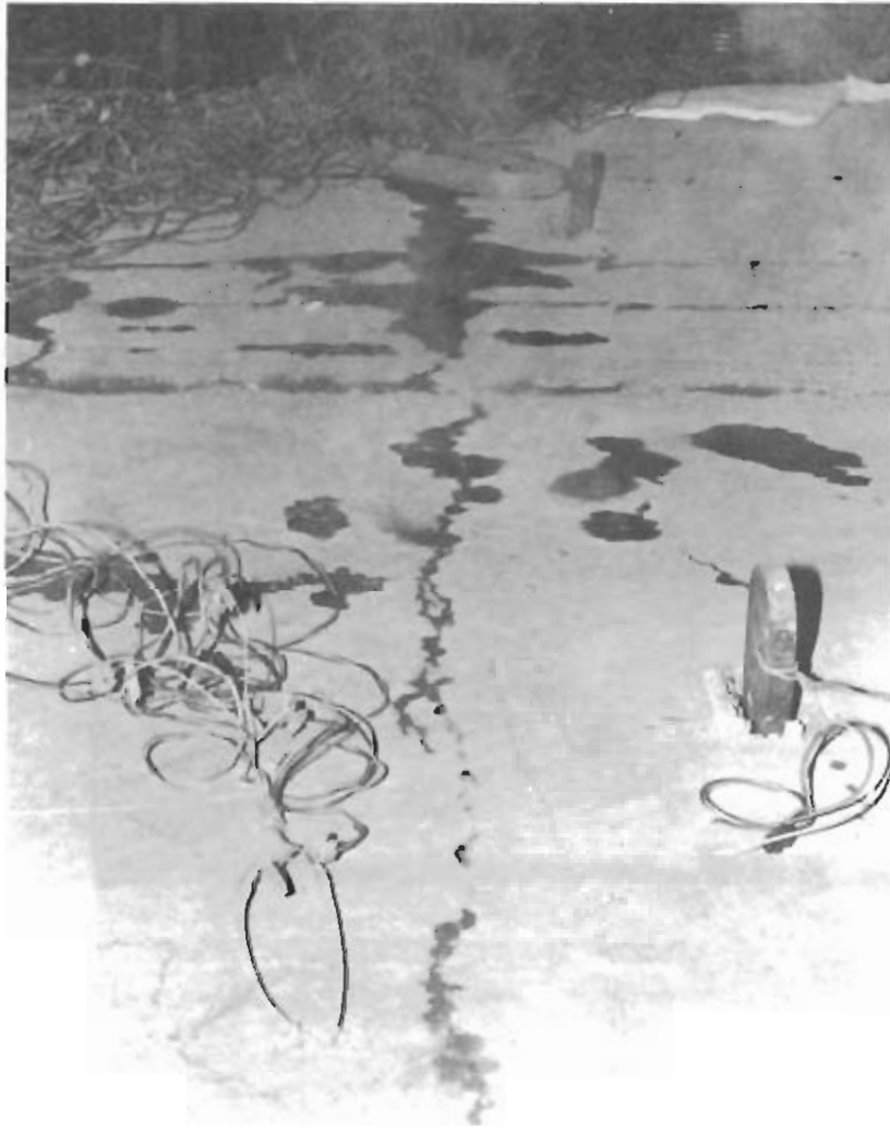
(a) Transverse hairline cracks
