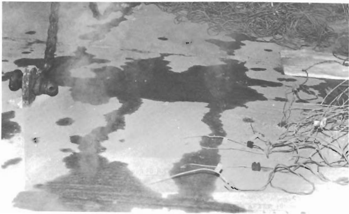
(b) Moisture on light-weight concrete slabs
